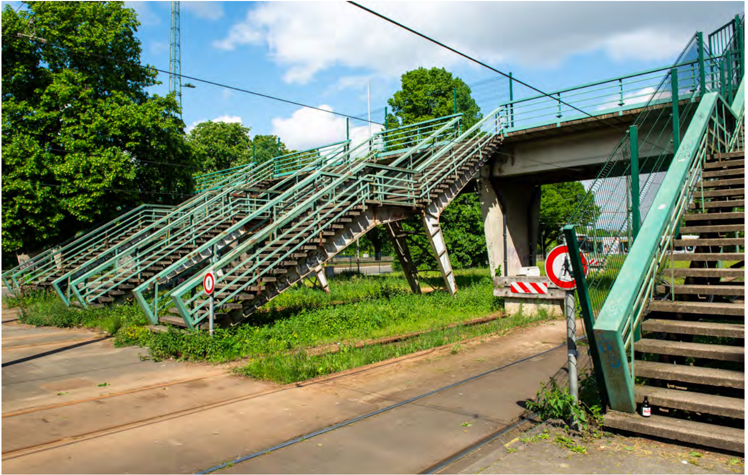
The staircases have been closed for several years due to their deteriorated condition (photo by author)
