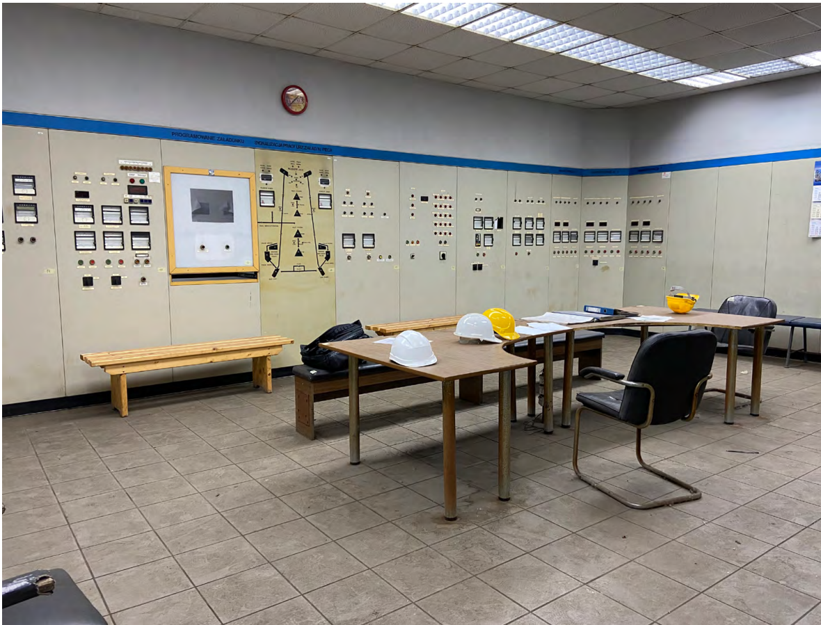
Interior of control room in 2023 (photo by author)
