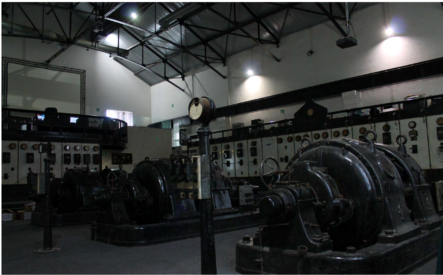
Siemens Schuckert Werke (SSW) turbogenerators inside the power plant (photo by author)
