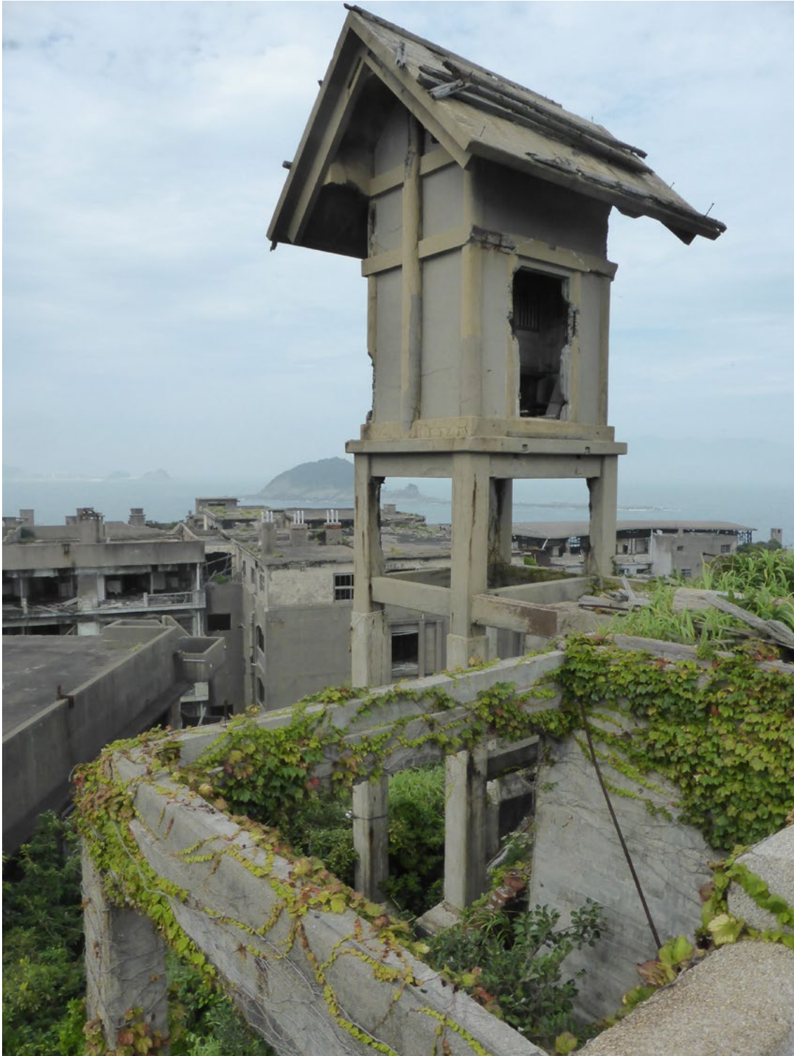
Due to a lack of proper maintenance since the mine closed in 1974, the buildings made of reinforced concrete, steel and wood have fallen apart or irreversibly decayed (photo by author)
