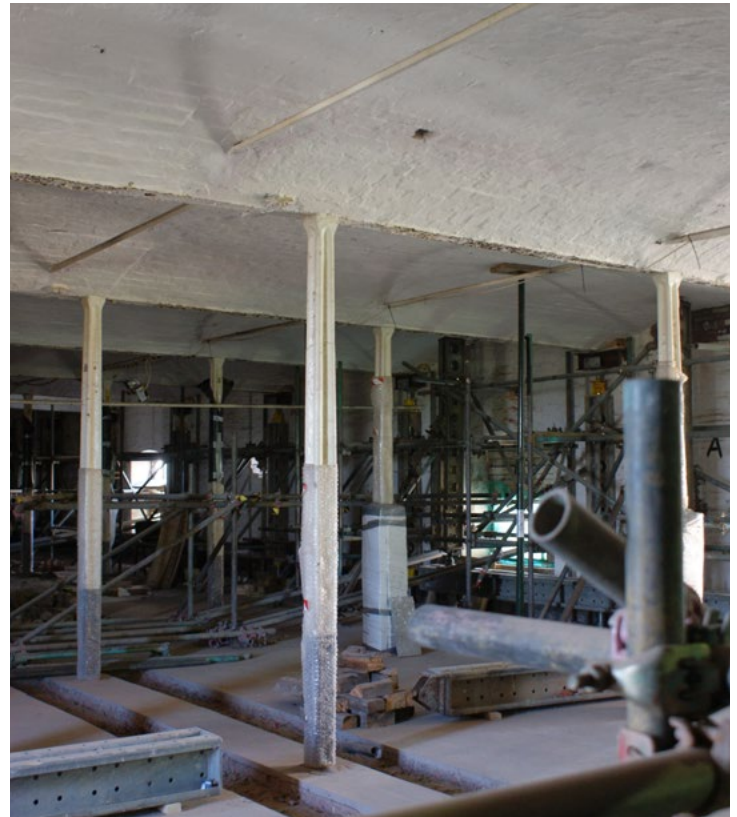
Shrewsbury flax mill, 1797, became a floor malting in 1897. A reinforced concrete mesh is being applied by Historic England over the original floor structure as a safety net, 2016 (photo by Mark Watson)
