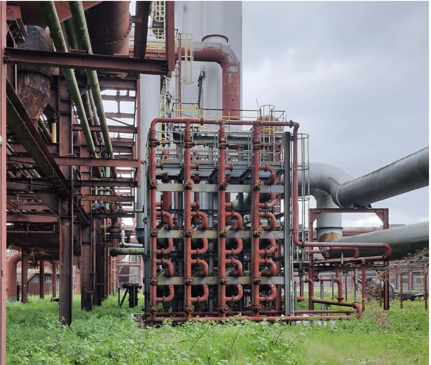
Industrial Heritage, heavily weathered: How to deal with it? Tubular coolers as part of the Ammonia-Washer in the coking plant of Zollverein. Photo: R Hillmann
