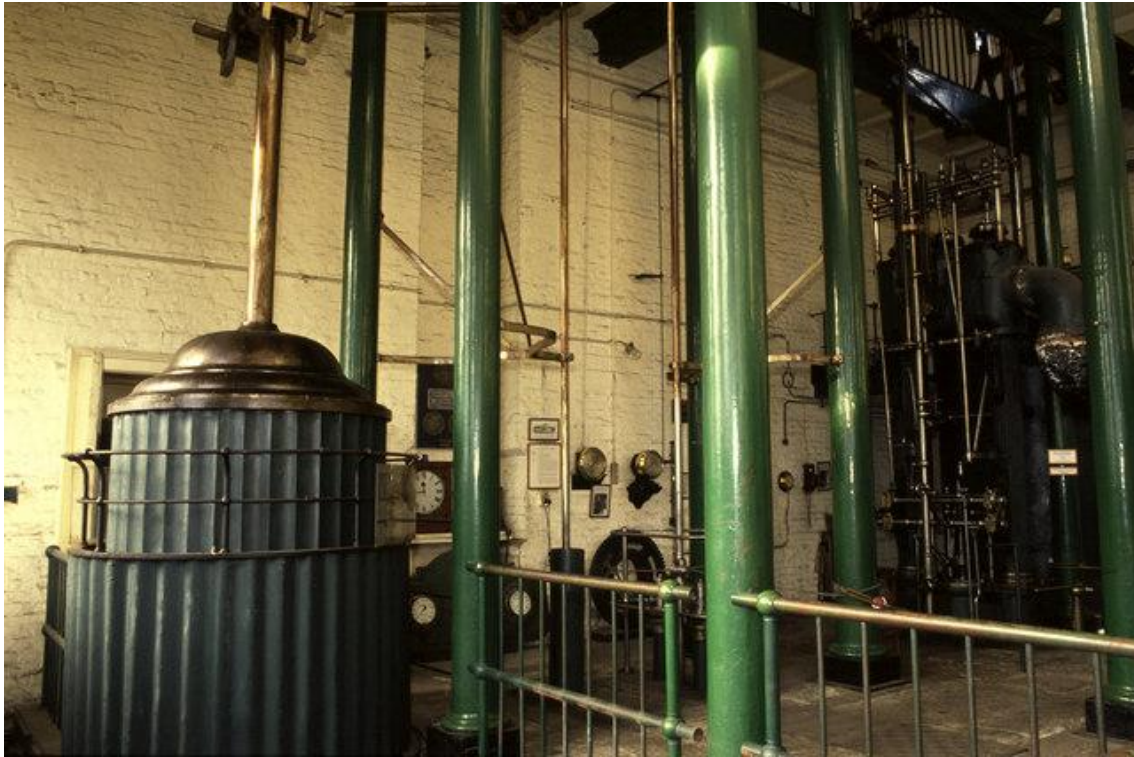
The 1820 Boulton & Watt beam engine, one of two originally installed at Chelsea Pumping Station beside the river Thames in London and moved upstream to the Kew Bridge pumping station in 1840. (Chris Allen, Creative Commons)
