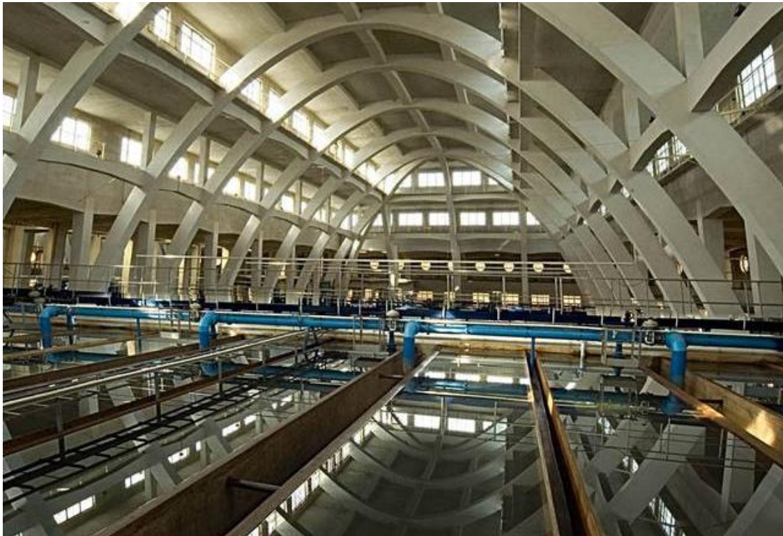
Parabolic concrete arches over the 1929 filter house of the Podolské treatment plant in Prague. (Prague Waterworks Museum)
