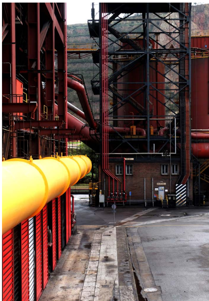
Aboño Thermal Power Station, decorated by the Asturian artist Joaquín Vaquero. The plant was built in 1974 and extended in 1985. It is an unusual generating plant, using fuel oil, diesel, coal from the coal mines of Asturias as well as imports, and the waste gases produced by the nearby Arcelor - Mittal Gijón steelmill.
