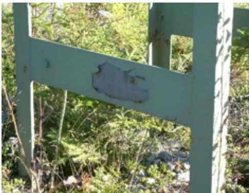
A 70-year-old coating starts flaking off
