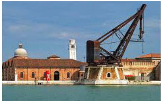
The Armstrong hydraulic crane in the Venice Arsenal was designed in 1893 to help service the ironclad warships of the Italian navy. The rivetted steel structure, rollers, rails and rotation platform, is suffering severe corrosion and needs urgent conservation treatment. -see Report on industrial rust
