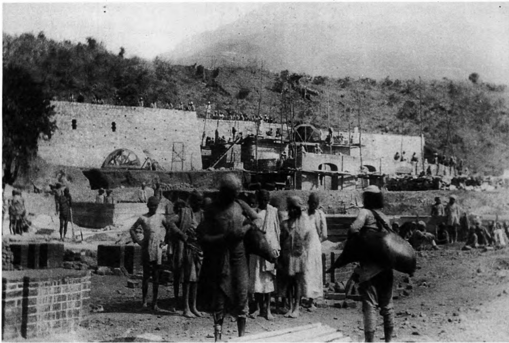
Figure 4. The new iron- and steel-works in Dechauri under construction in early 1863. The number of workers engaged at the site was up to 2,000. Photo: Gustaf Wittenström, National Museum of Science and Technology, Stockholm, C15057.
