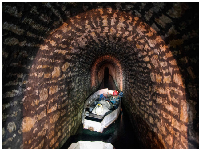
Friedrich Deep Adit, close masonry arched tunnel lining, typical of a great many kilometres that still function in the purpose for which they were constructed almost two centuries ago.
