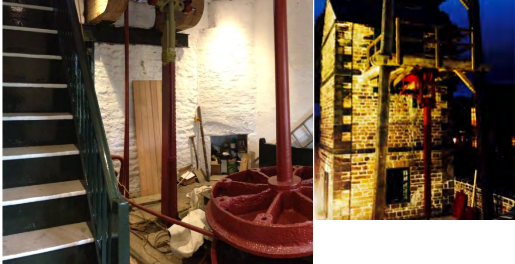
Elsecar pumping engine near Barnsley, the piston ready to go back into the cylinder. © Industrial Heritage Consulting Ltd
