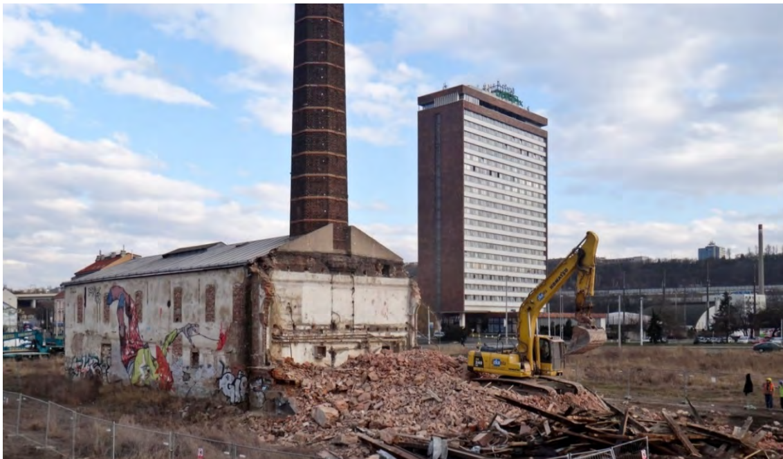
Among the most talked about demolitions in recent years was the destruction of the boiler house of strojírny Rustonka, one of the symbolic reminders of the early stages of the industrial age in Prague. © Jan Zikmund, 2014
