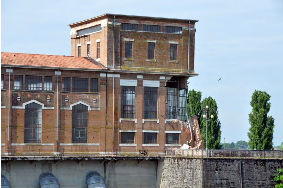
The Mondine Water Plant after the earthquake. © Arlotti G., 2013
