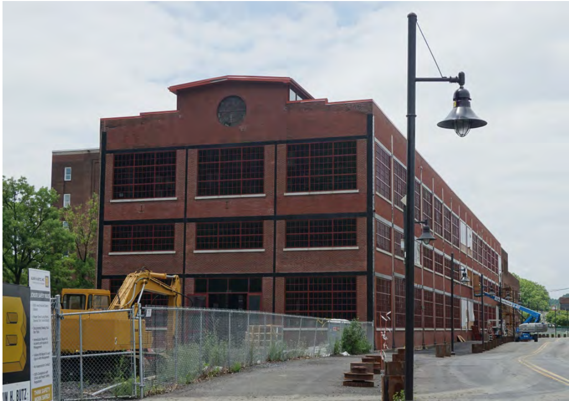
Construction of the National Museum of Industrial History underway in Bethlehem, Pennsylvania. © Bode Morin, 2015
