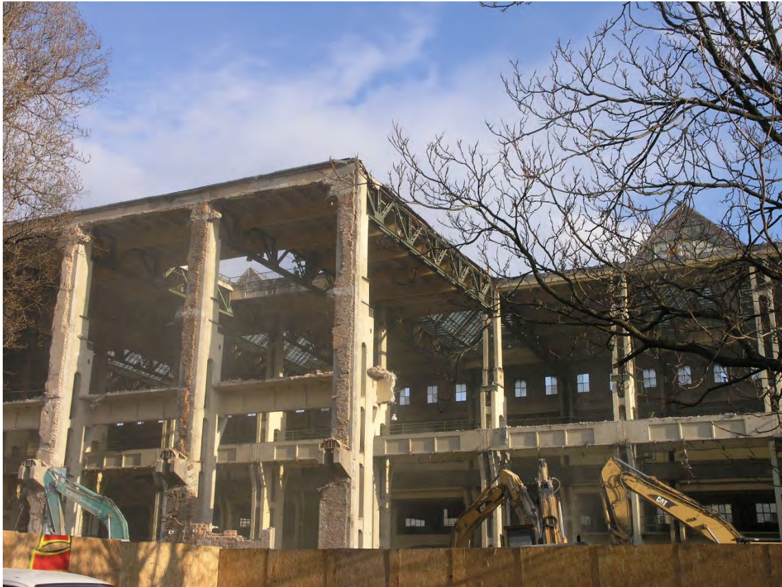
Demolition of the monumental hall of the former Ganz electric works in Budapest. (Photo: Györgyi Németh, 2015)
