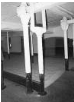
The cast-iron columns and capitals for running the line shafting bearing the wide jack-arch floor. Photo: Shropshire Archives
