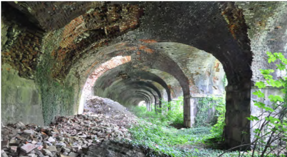
Inside the gallery: stones have fallen, bricks of the vault are flaking and sections of the gallery even broke down.
