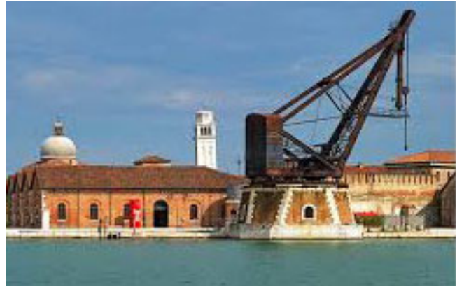
The Armstrong hydraulic crane in the Venice Arsenal was designed in 1893 to help service the ironclad warships of the Italian navy. The rivetted steel structure, rollers, rails and rotation platform, is suffering severe corrosion and needs urgent conservation treatment. -see Report on industrial rust
