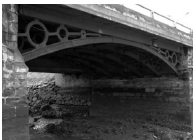
The re-used spans of the Bilbao bridge over the river Udondo at Lejona
